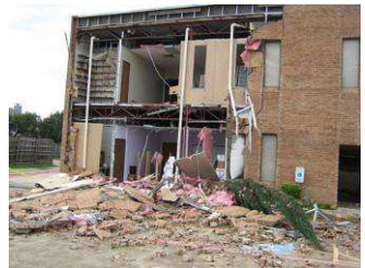
Above: Tornado damage here in Carrollton, TX
